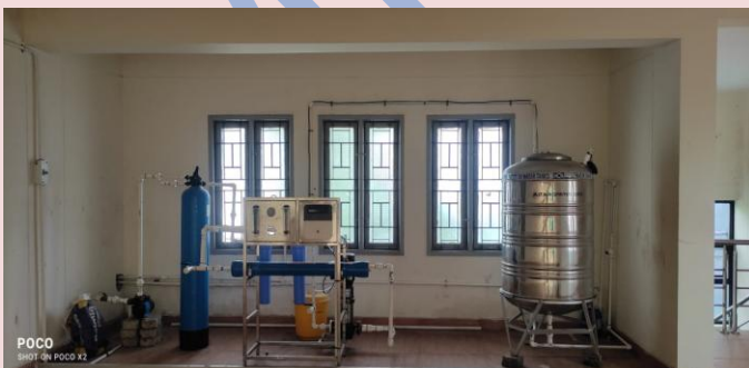
RO Water Plant
