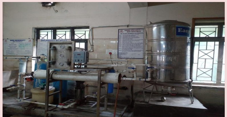
RO Water Plant
