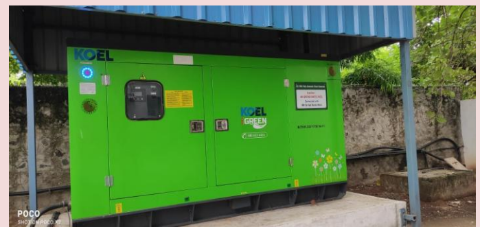
24 X 7 Power Backup (DG Set)
