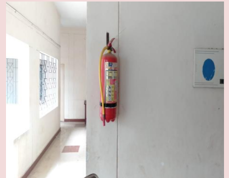
Fire Fighting Extinguisher
