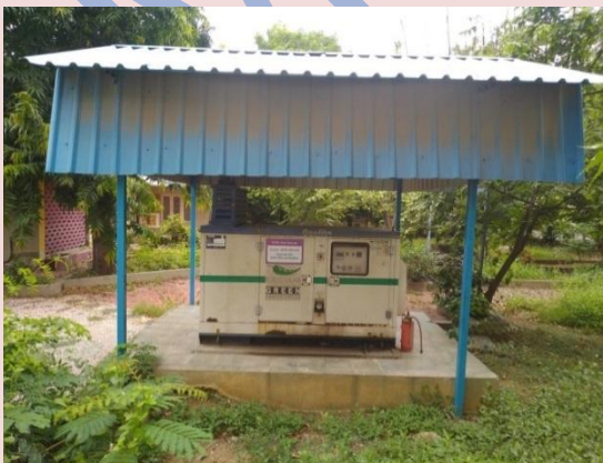
24 x7 Power Backup (Diesel Generator)
